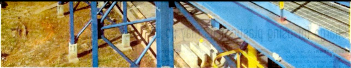
Under the new standard operating procedure, a 700m conveyor system will transport bauxite directly to the ship. PIC COURTESY OF KUANTAN PORT
